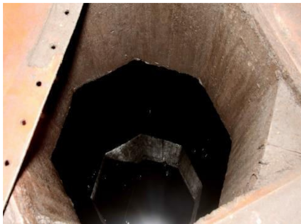
Fig 4 B: Man-whole of contaminated PCB oil with direct leachate into the Lagoon
